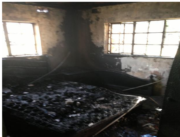
Pic.2 House Fire
